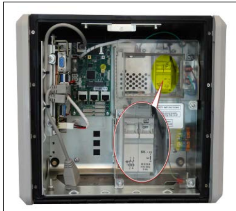
Figure 5-34: Main Power Switch - OFF
