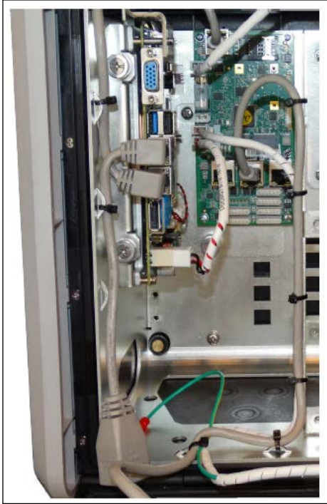
Figure 5-37: Connected to CommBoard
