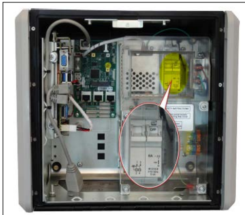
Figure 5-25: Main Power Switch - OFF
