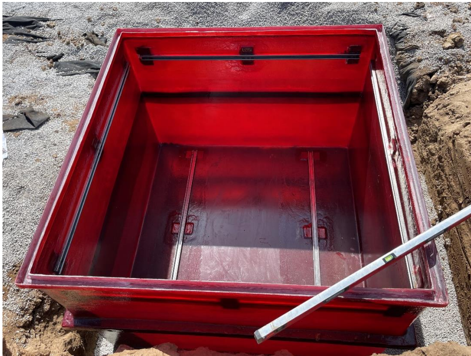
Figure 8: Typical Underground Installation Sump
