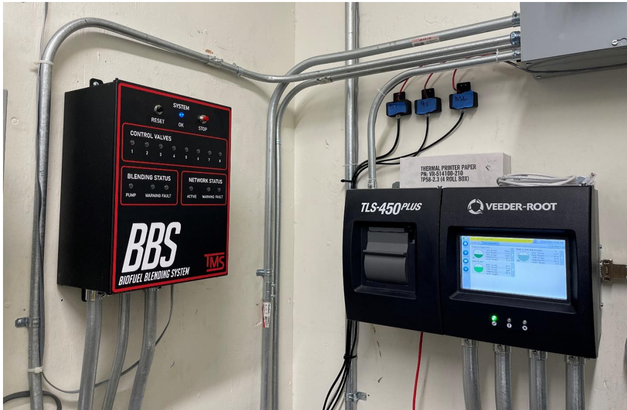
Figure 17: Typical mounting of BBS control panel in the back office
